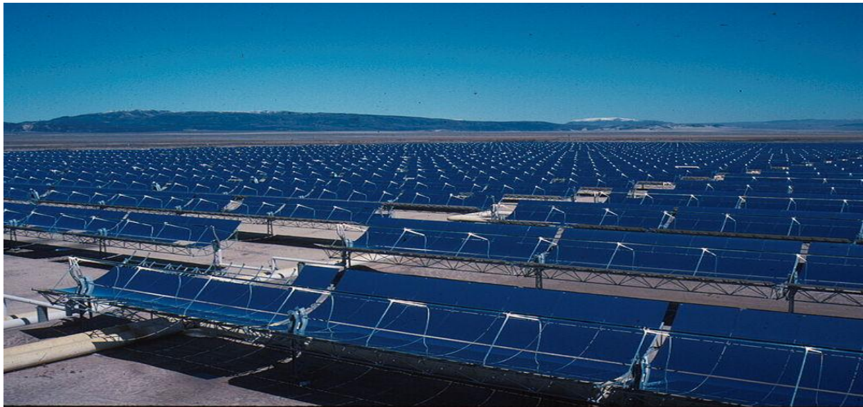
Figure 3.7 The 354 MW SEGS solar complex in San Bernardino, California, USA.
