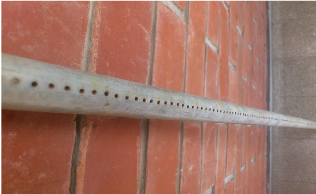
Fig. 3.3: Pipe for Spraying Water
