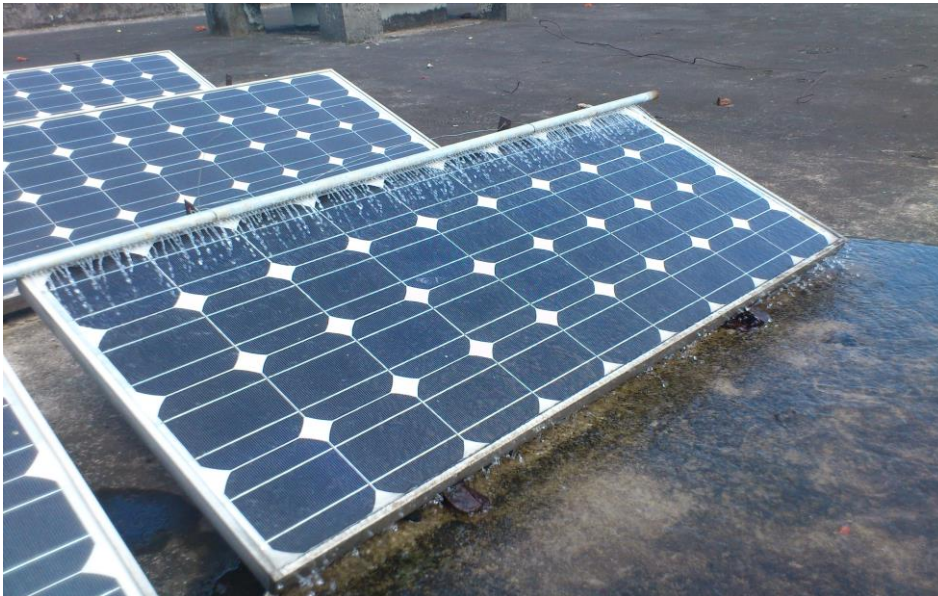
Fig. 3.5: Installed setup in IUT Campus
