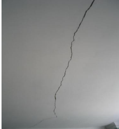
Fig.1.2 A wall crack
