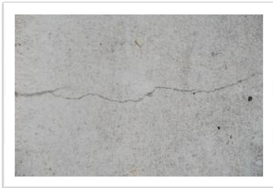
Fig. 3.1 Original Image of a cracked surface
