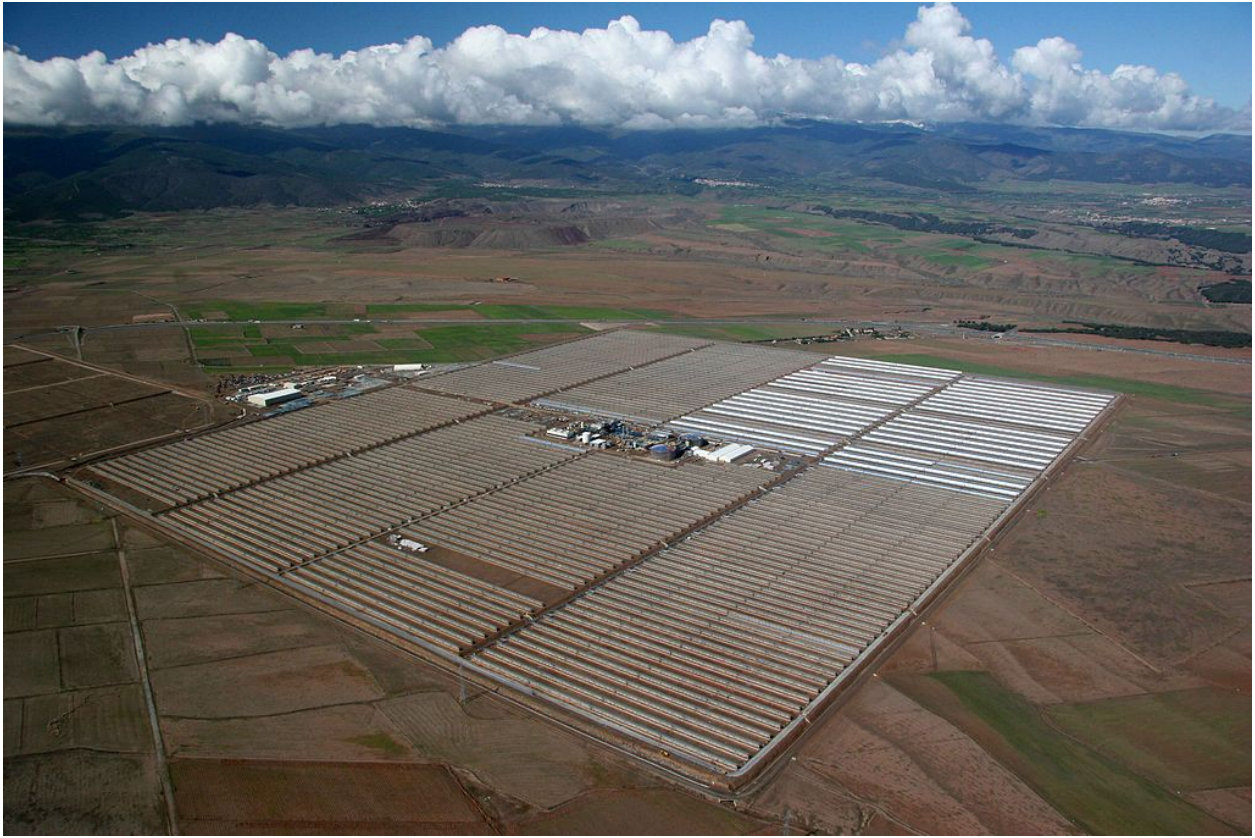
Fig.1. the 150 mw Anda sol solar power station
