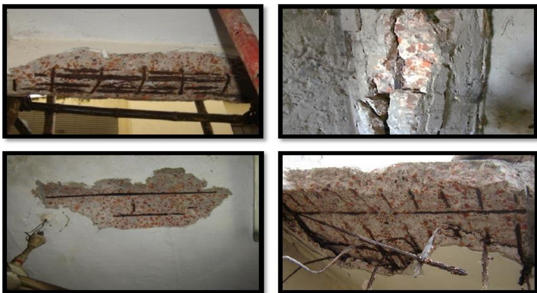
Photo 1.1: Corrosion of steel due to Carbonation: structures in Dhaka city.
