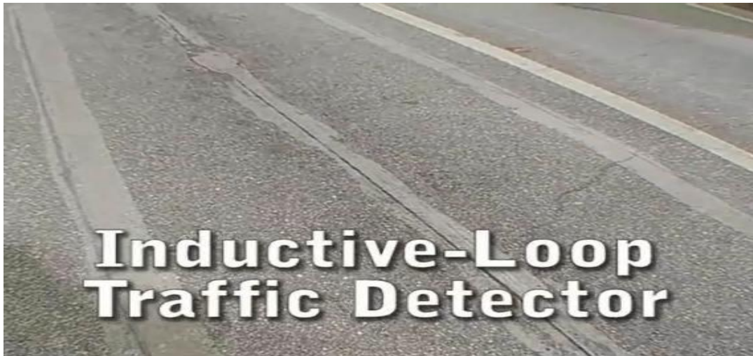
Figure 18: Inductive loop sensor on the road
