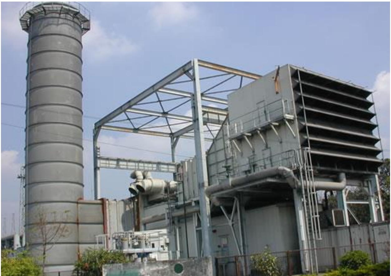
Figure 5: Tongi 80MW Power Plant
