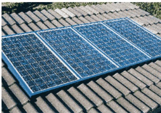
Solar panels mounted on a tilted roof.
