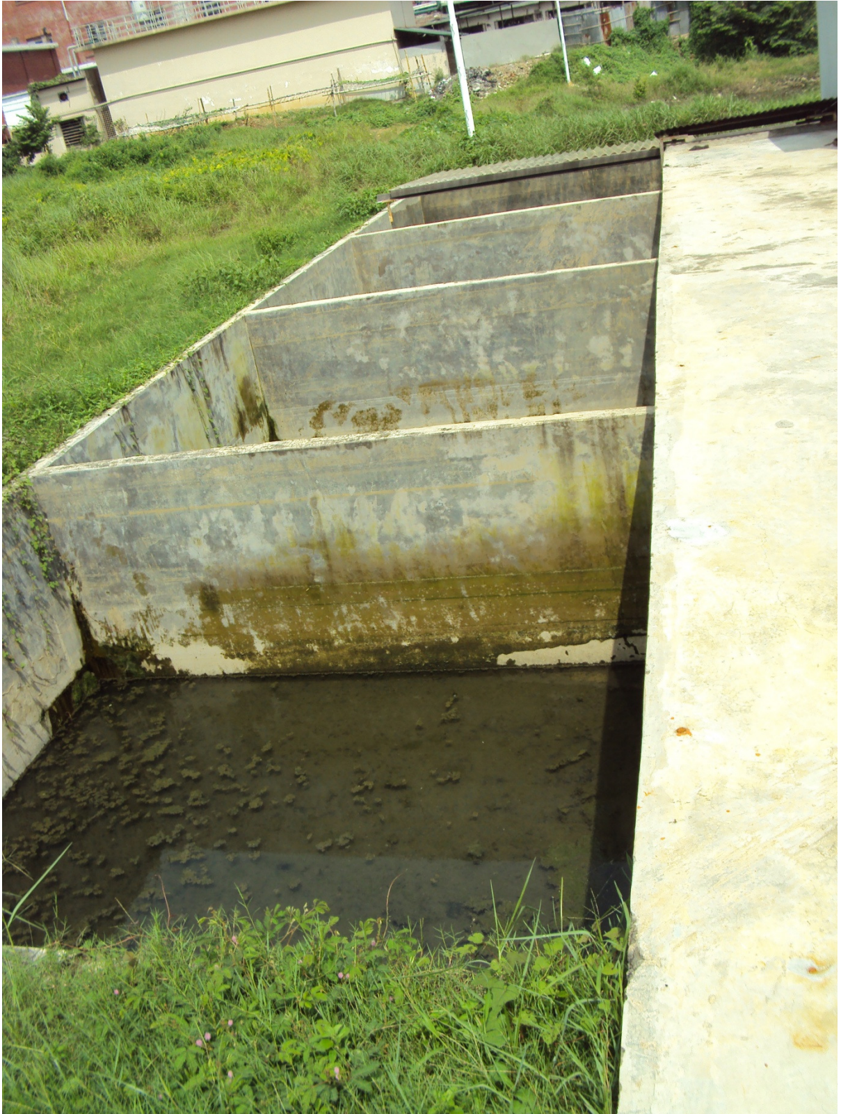
Photo 4.12: Sludge Drying Beds in CETP
