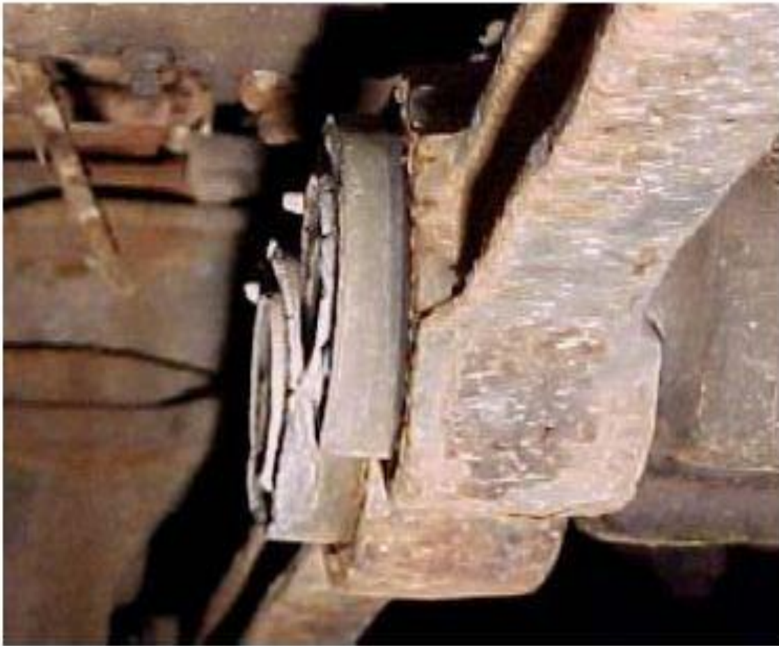
Figure 9. The outer metal sleeve has completely separated from the rubber on both of the above rod ends, allowing the torque rods to slide against the frame.
