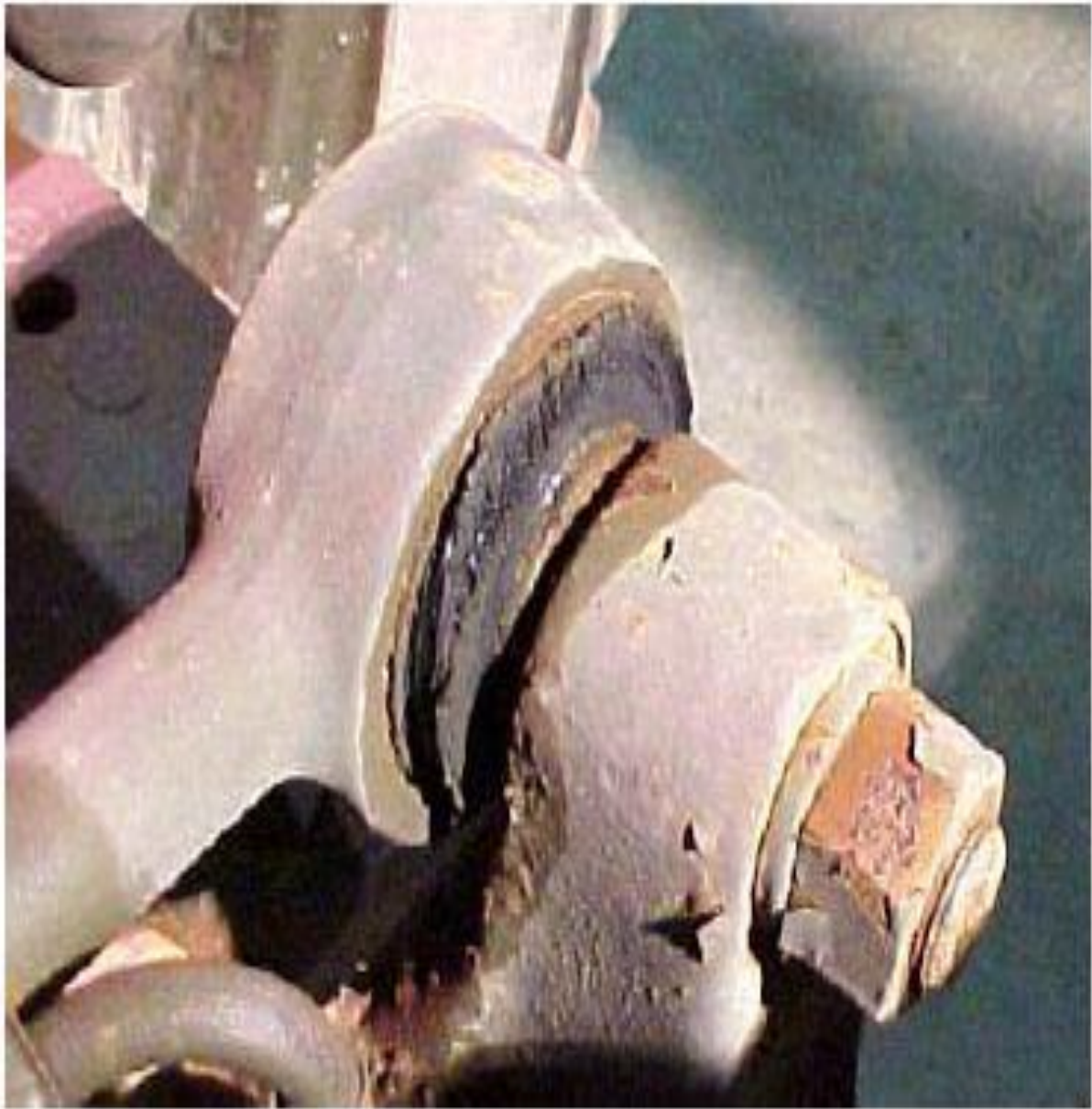
Figure 11. This is an example of the rubber separating from the outer metal sleeve of the ball joint. This rod end should be replaced.
