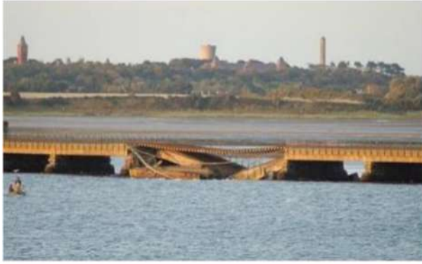
Figure 2: Bridge failure due to scouring effect
