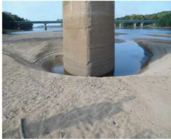
Figure 1: Scouring effect around a bridge pier[16]
