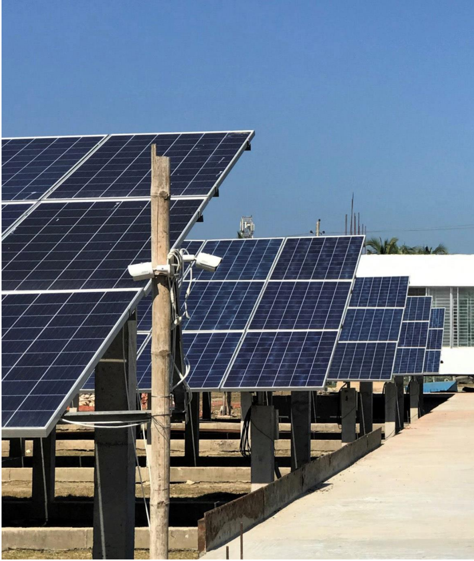
Figure 6: Currently operational PV plant in St. Martin's Island
