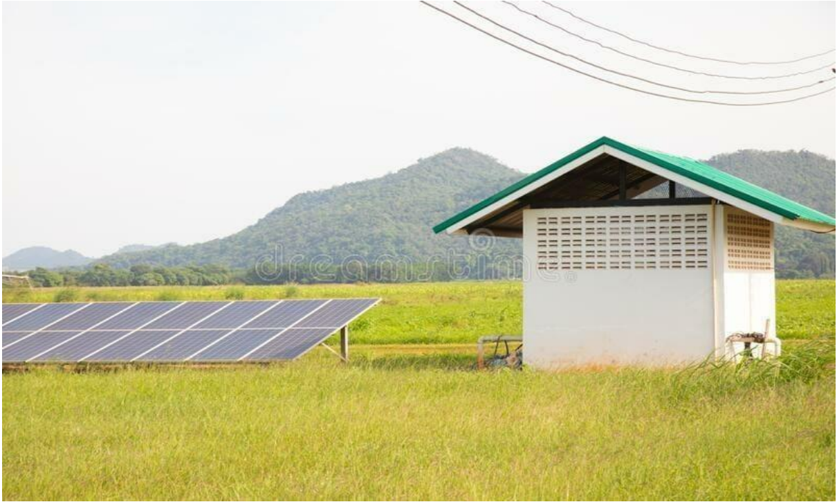
Figure 4: Solar Cell in a remote location
