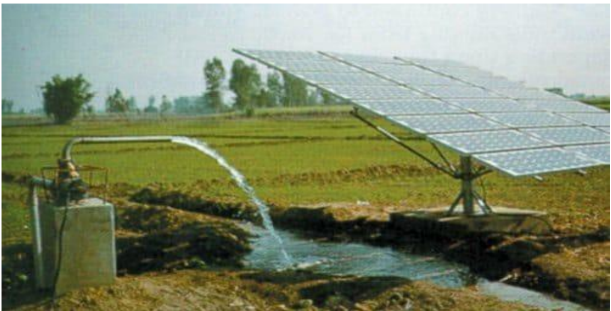
Figure 5: Solar Cell for water irrigation pump
