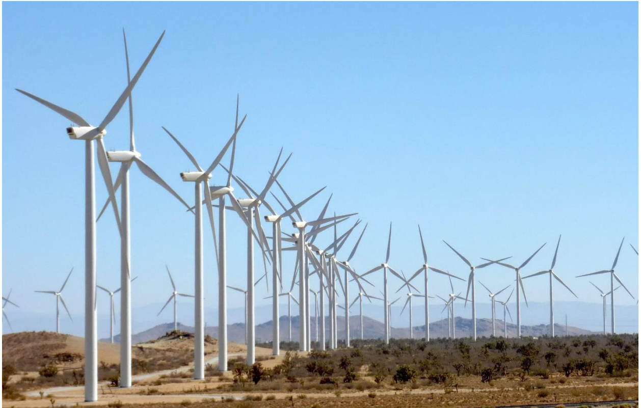
Figure 30: Alta Wind Energy Centre
