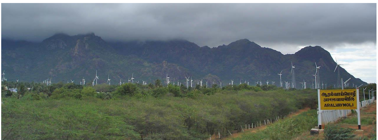
Figure 31: Muppandal Wind Power Plant
