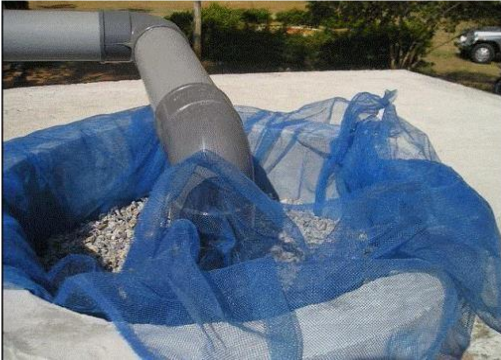
Figure 3: Photograph of Typical Filter in Rainwater Harvesting
