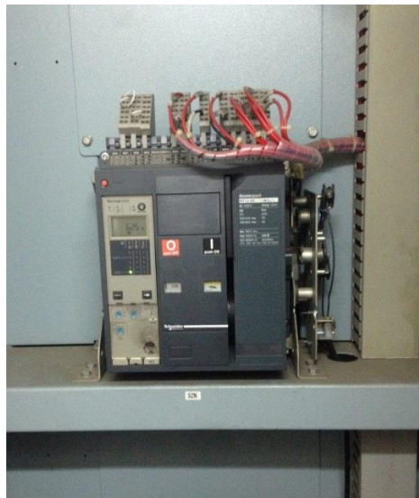
Image: One of the Circuit Breakers in the IUT Substation
