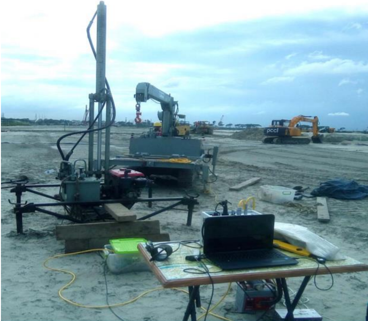
Figure 3.1.2: Field Setup of Geomil Equipment Fox 100 CPTU Image Source: Prosoil Foundation Consultant
