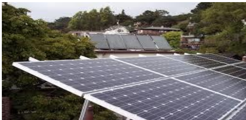
Figure 7: Solar Panels on rooftop
