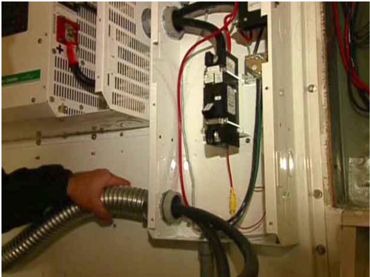
Fig 2.5.2 Interior Electrical Connections
