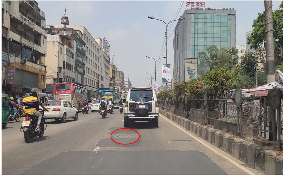
Figure 4-14: Pothole After flyover before Shainik Club
