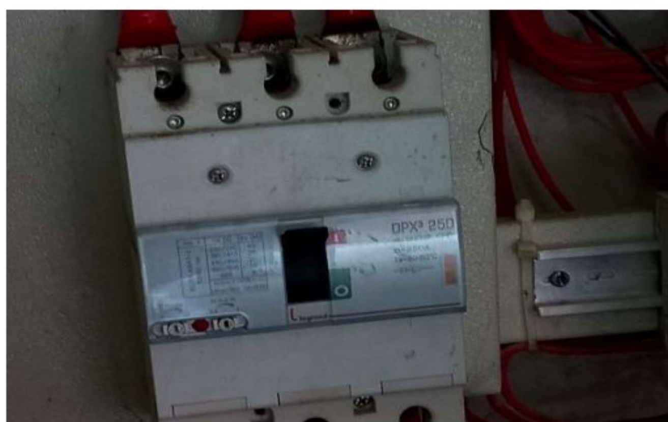
Figure 4.31: The 250 A MCCB (TP) breaker that comes from the main busbar of the LT panel to the distribution boxes for light loads like tube-light, fan etc.
