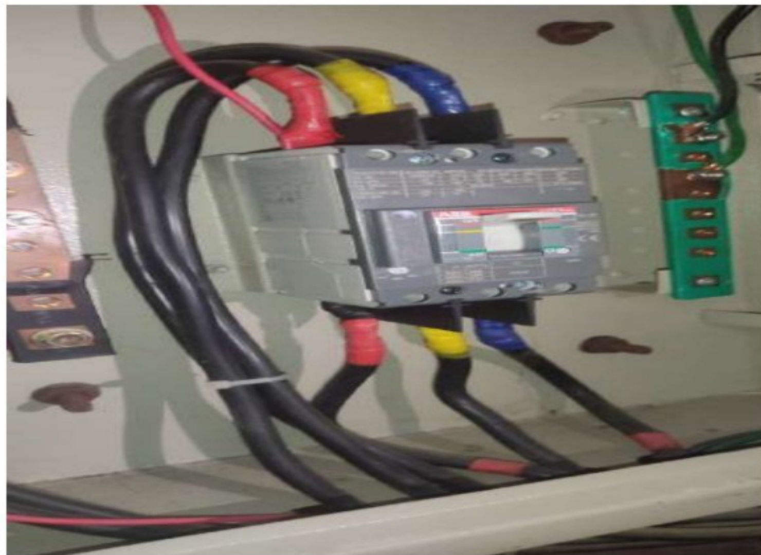
Figure 4.12: 160 A (TP) MCCB circuit breaker that comes directly from LT panel that goes to the lift of first academic building
