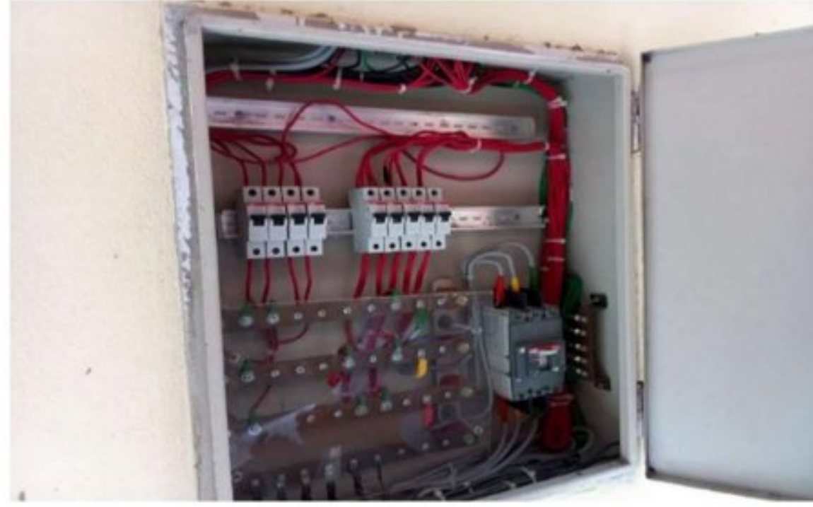
Figure 4.35: Sub distribution box (that goes to each room of 3rd academic building)
