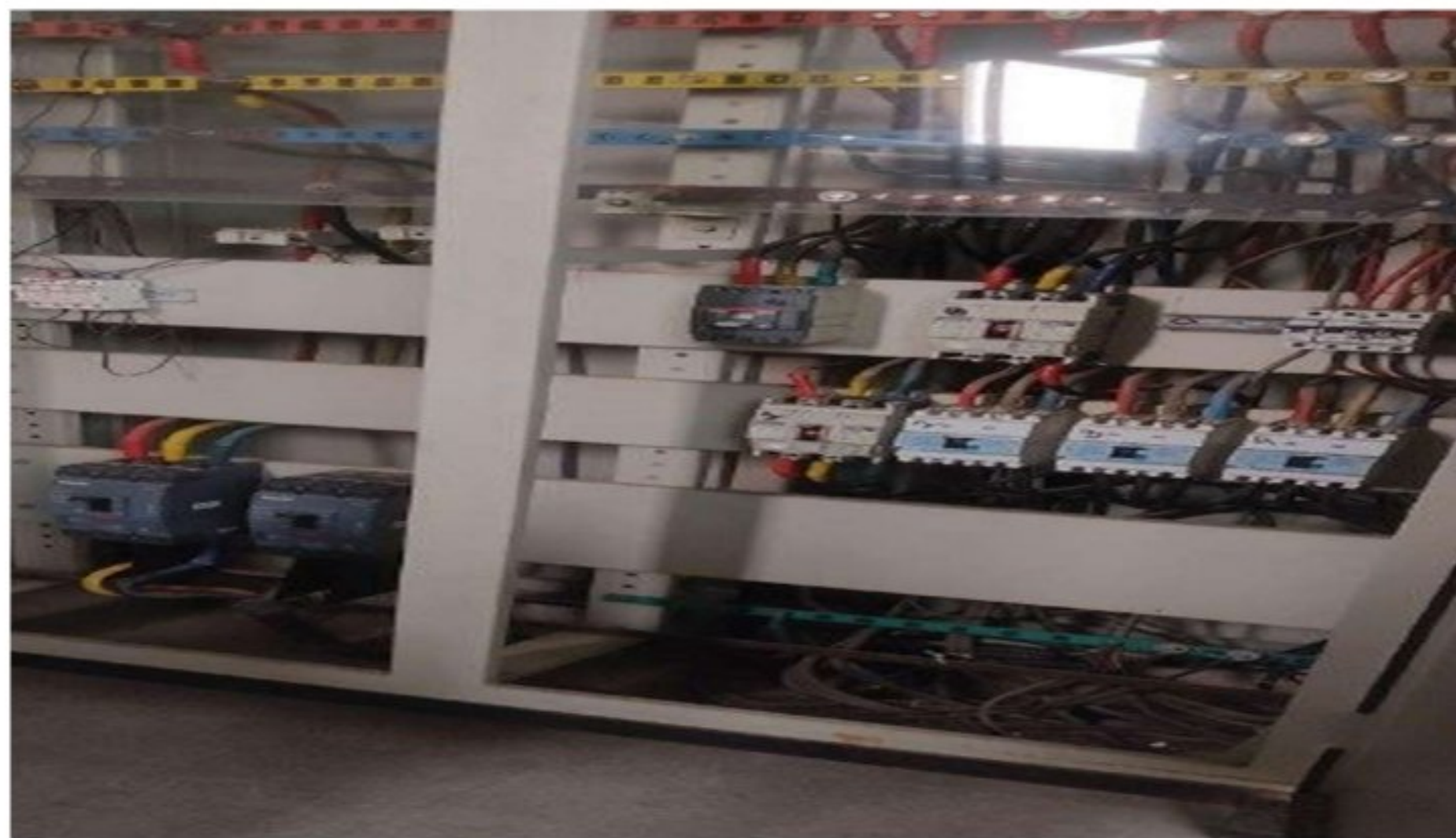
Figure 4.13: Main distribution board from LT panel situated at the ground floor of first academic building
