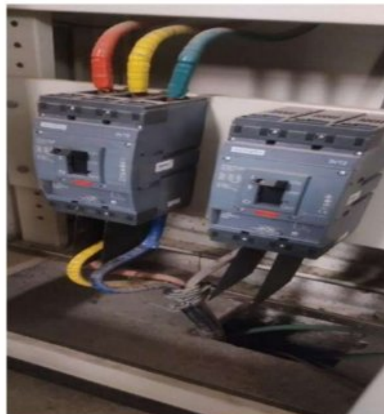
Figure 4.14: Main MCCB (TP) breaker coming from the LT panel to 1st academic building
