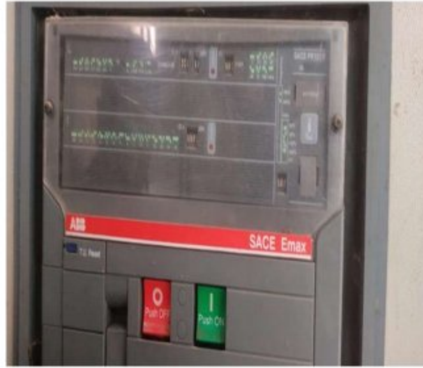
Figure 4.22: Main breaker that is coming from the LT panel to the second academic building that is a modified breaker tuned to 500 A for convenience of rating required
