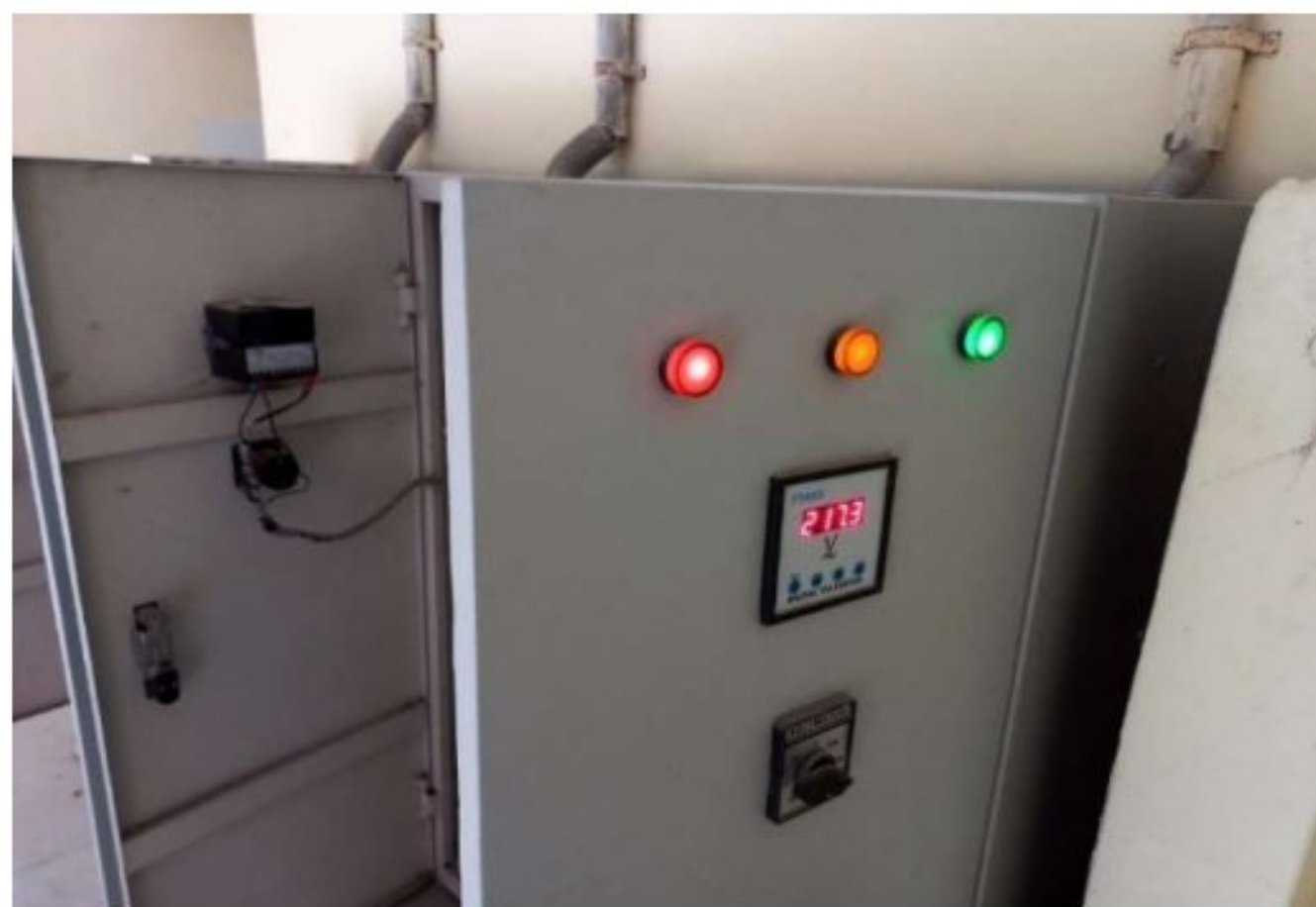
Figure 4.34: Voltmeter assigned to the main distribution board for the loads for constant maintenance of the upcoming voltage from the LT panel
