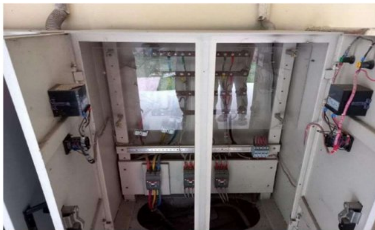
Figure 4.30: Main Distribution board of the 3rd academic building that goes to heavy load of each rooms like air-conditioner
