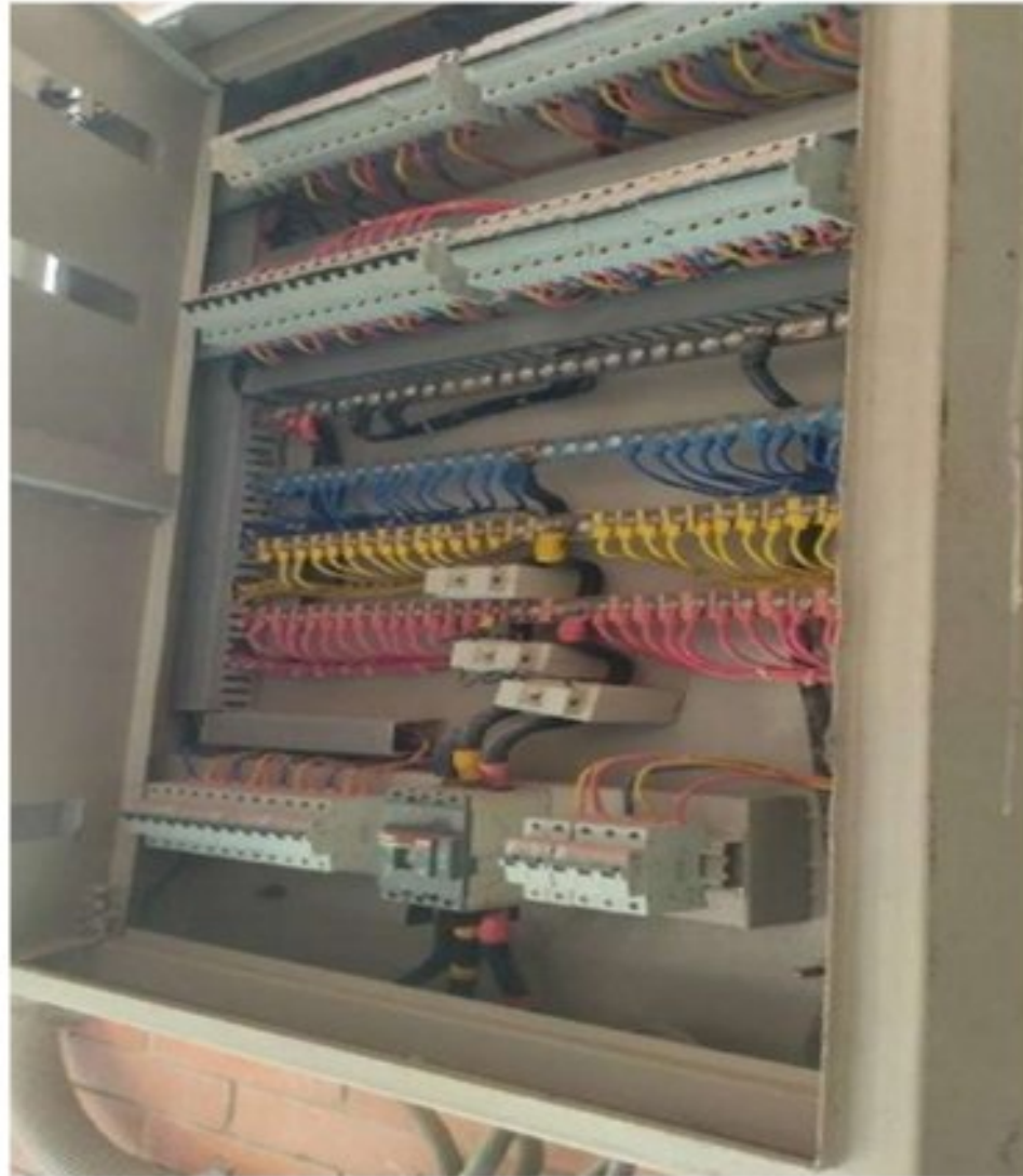
Figure 4.25: Main distribution board of second floor (and third floor) also of 2nd academic building (only for AC load)
