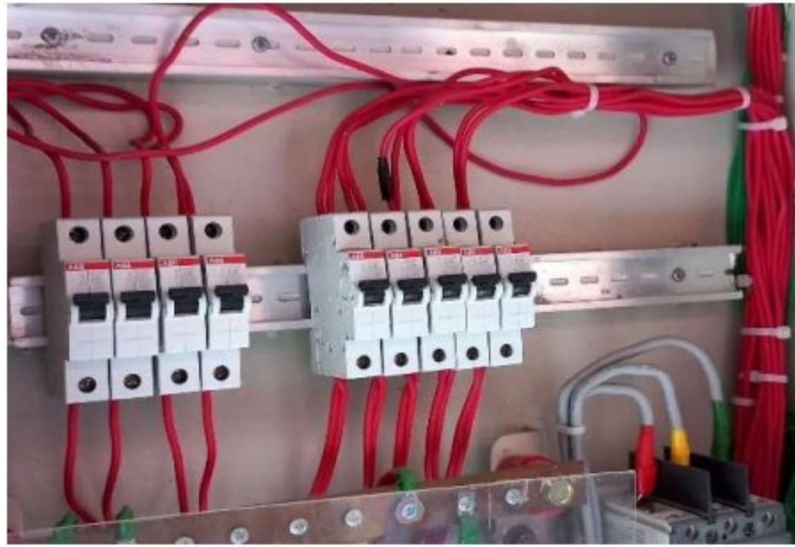
Figure 4.36: 10 A MCB (SP) circuit breakers that protects each room of the 3rd academic building
