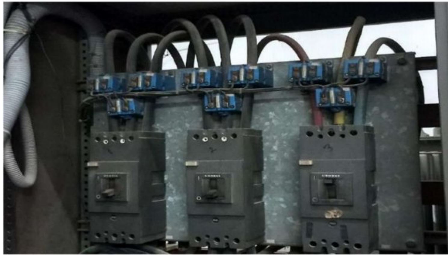
Figure 4.11: Circuit Breakers from main busbar of LT panel that goes to 1 st academic building
