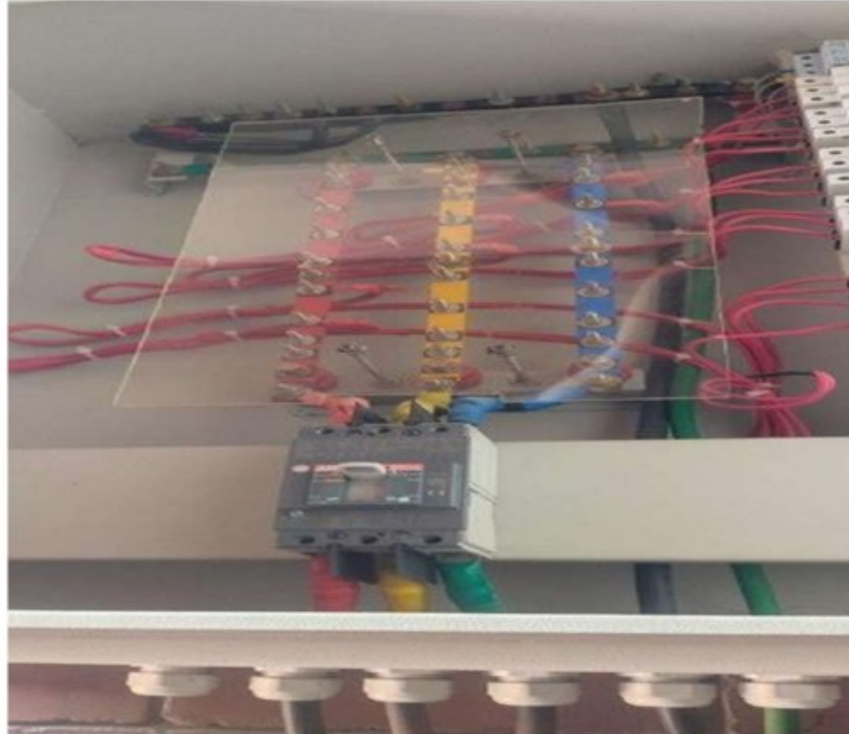
Figure 4.18: Main distribution board (AC load) of 2nd floor of 1st academic building
