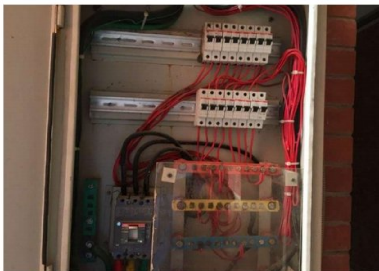
Figure 4.20: Main distribution board (AC load) of 4th floor of 1st academic building
