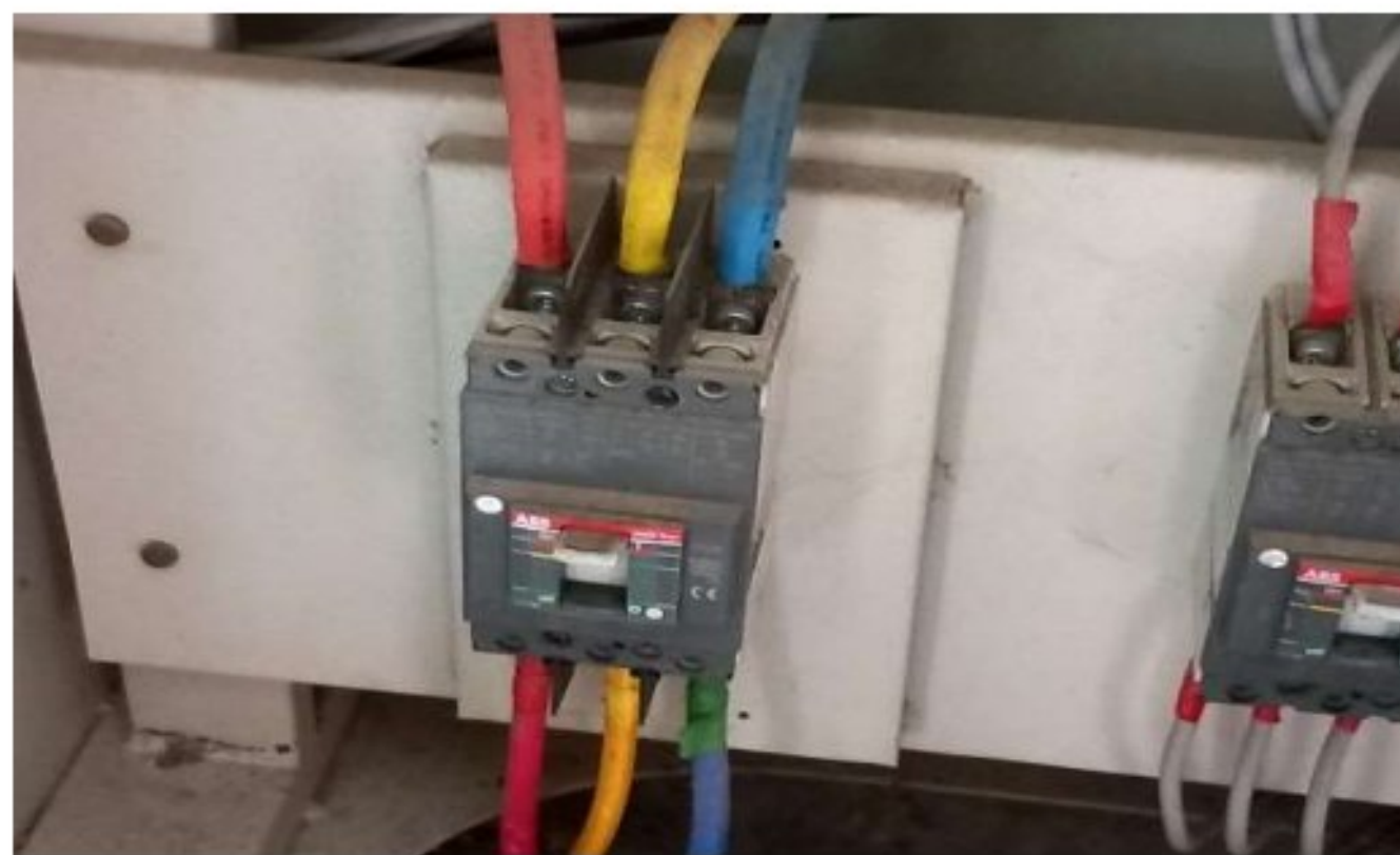
Figure 4.33: The 250 A MCCB (TP) breaker that comes from the main busbar of the LT panel to the distribution boxes for heavy loads like air conditioner.
