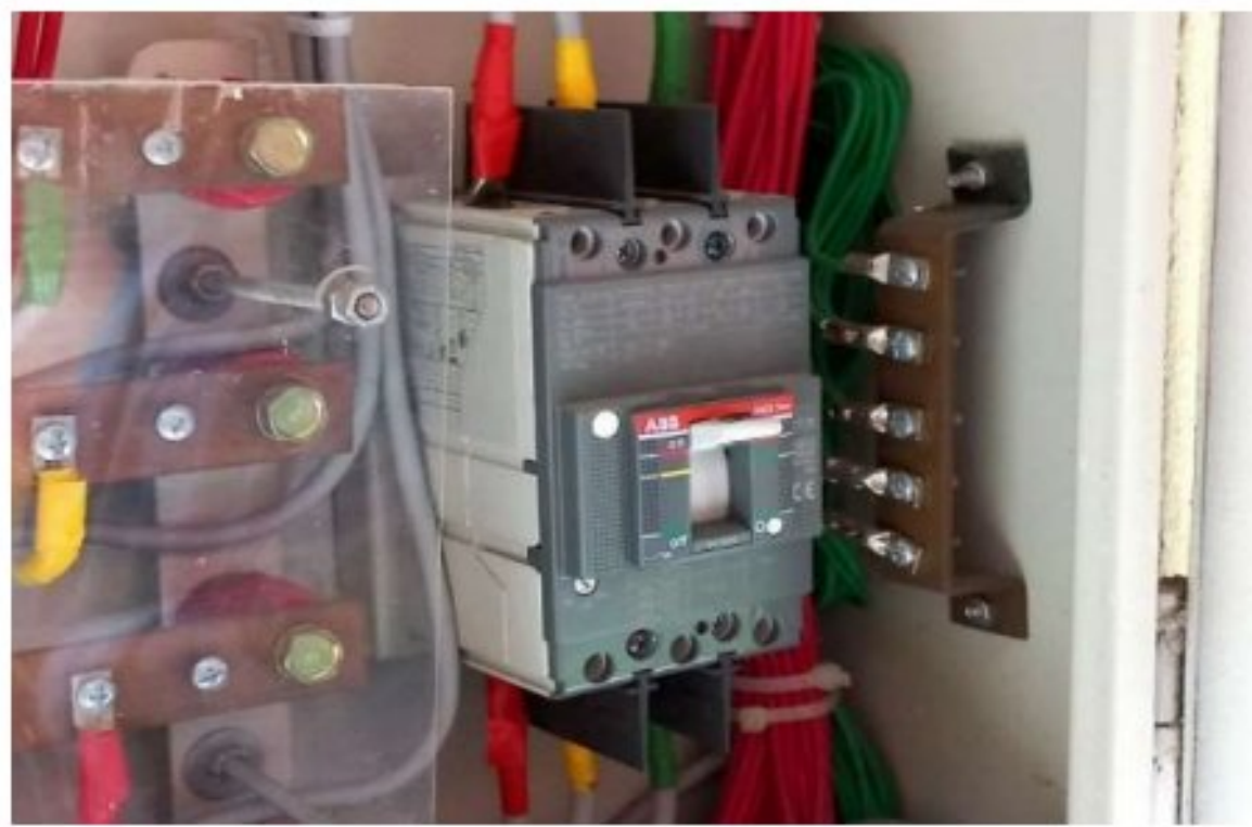
Figure 4.37: The 160 A MCCB (TP) breaker that is used on the sub distribution board of the 3rd academic building
