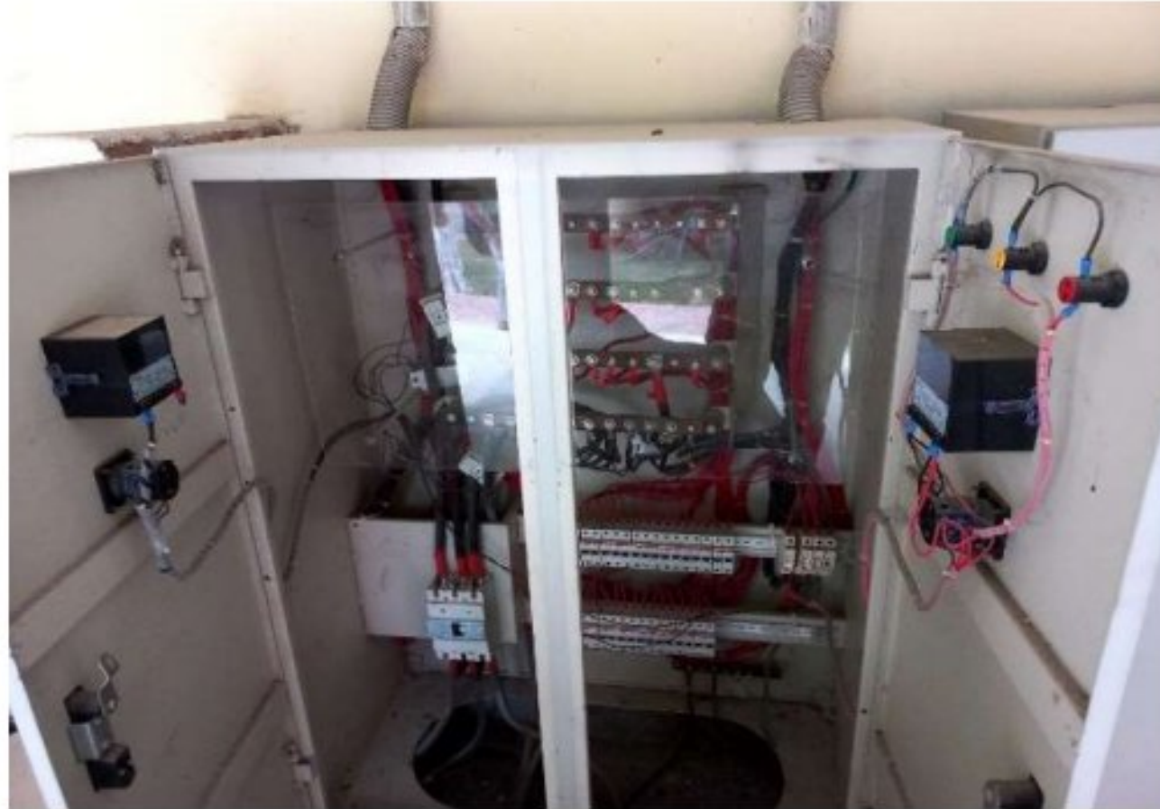
Figure 4.29: Main Distribution board of the 3rd academic building that goes to light loads of each rooms like tube-light, fan etc.
