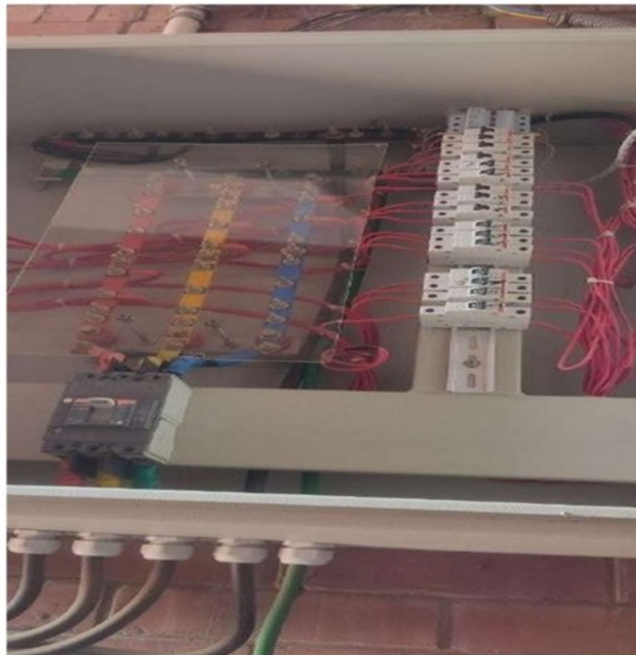
Figure 4.17: Main distribution board (AC load) of 1st floor of 1st academic building
