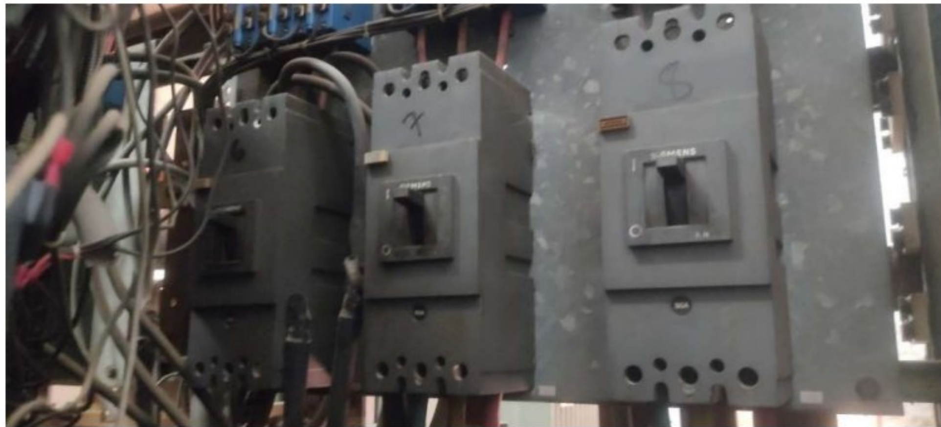
Figure 4.9: Circuit Breakers from main busbar of LT panel that goes to 1 st academic building
