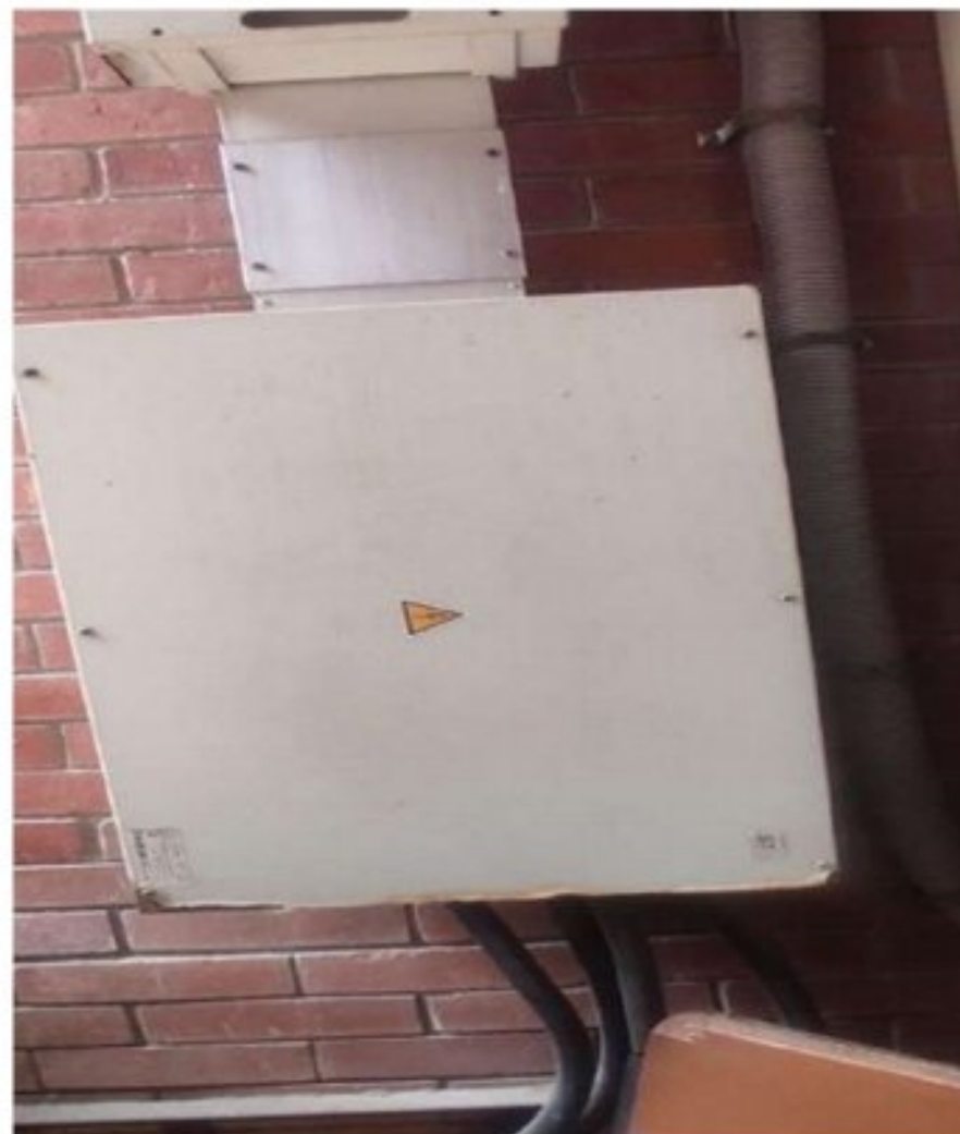
Figure 4.24: Busbar Trunking System (BBT) of second floor of second academic building (BBT also present on other floors as well) with circuit breaker mounted on this special busbar
