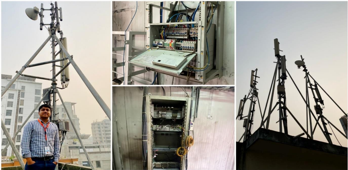
Figure 26: BTS (Base Transceiver Station) Audit and Visit - Antena
