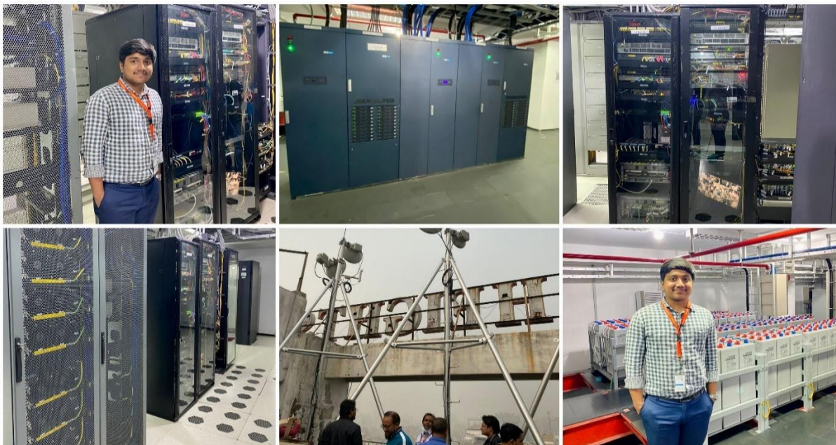
Figure 25: MSC (Mobile Switching Center) Audit and Visit
