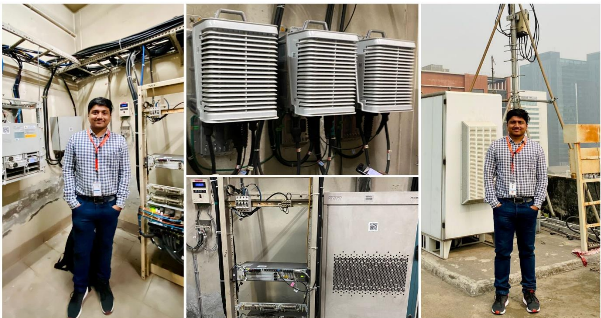
Figure 27: BTS (Base Transceiver Station) Audit and Visit - Rectifier
