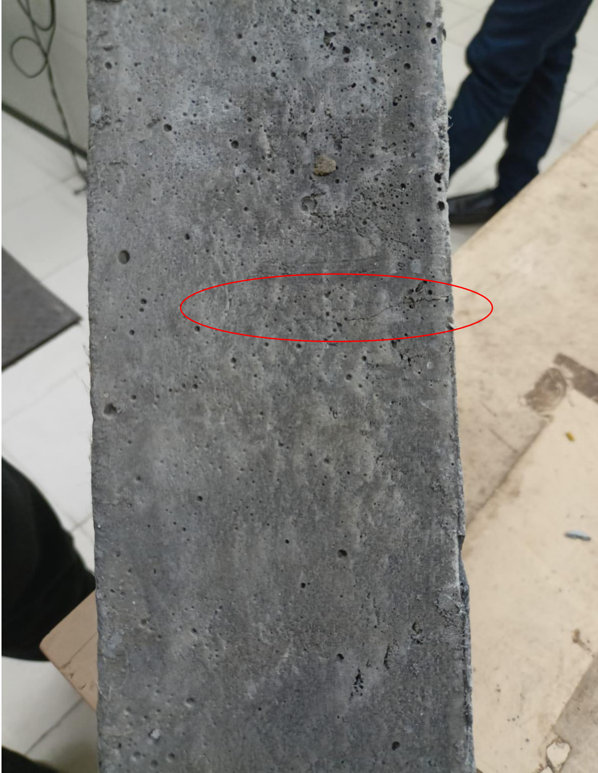
Figure 20: Failed beam sample from 2nd batch.
