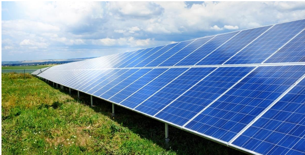
Figure 4.8 Solar PV Array.
