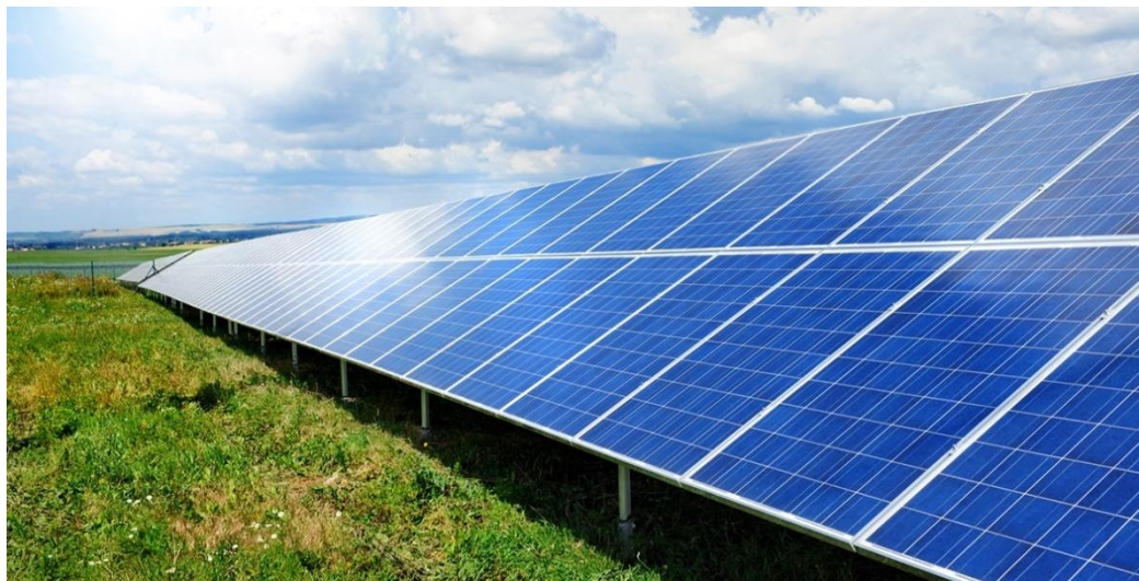
56. Figure 4.8 Solar PV Array.
