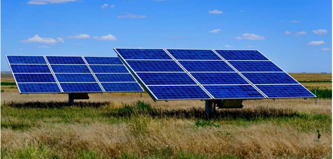
Fig 2: A view of Solar panels
