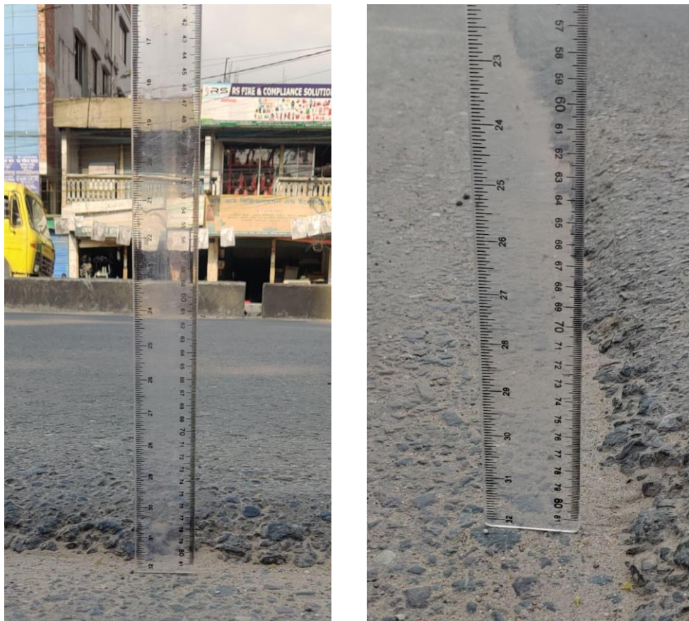
Figure 10: Shoulder Drop-off in Location 01 (Using t-scale)
