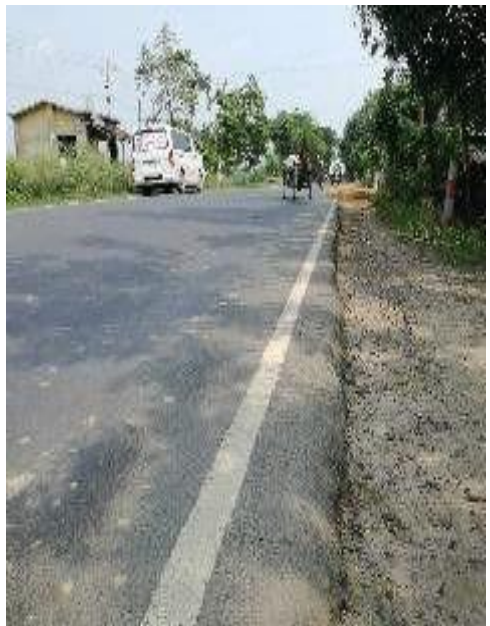
Figure 3: Risky & Defective Shoulders
