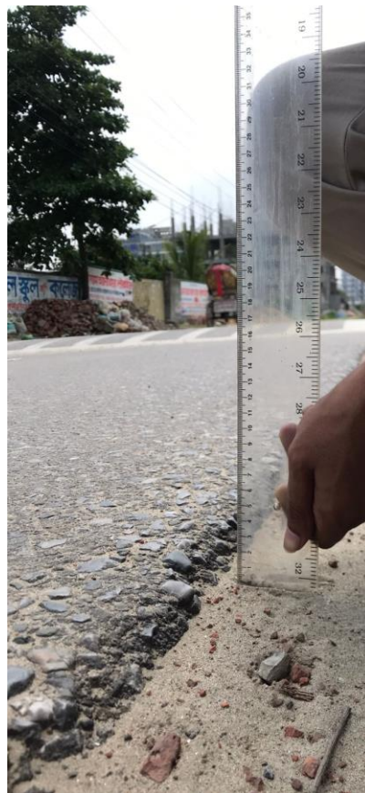
Figure 16: Shoulder Drop-off in Location 03 (Using t-scale)
