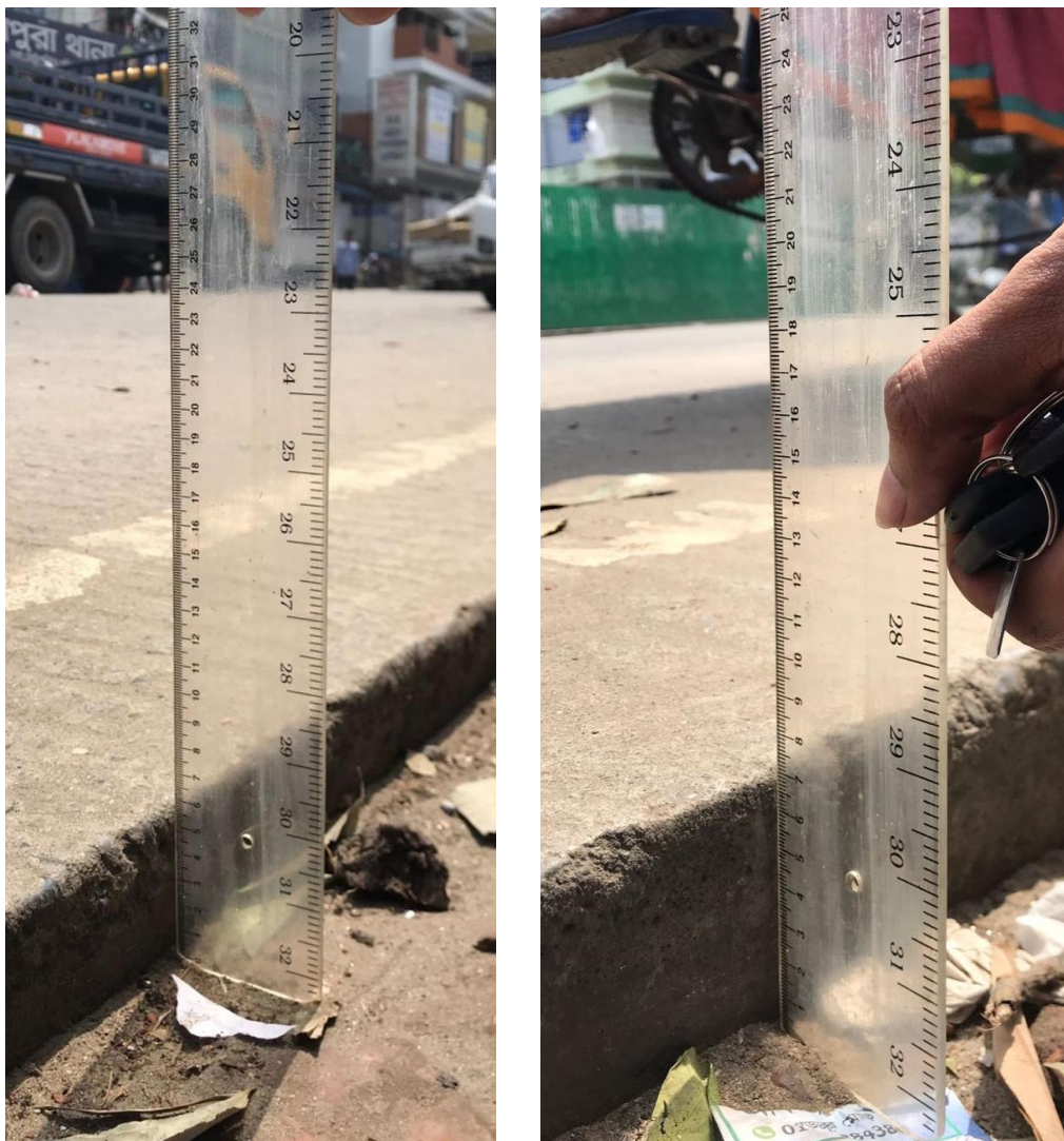
Figure 13: Shoulder Drop-off in Location 02 (Using t-scale)
