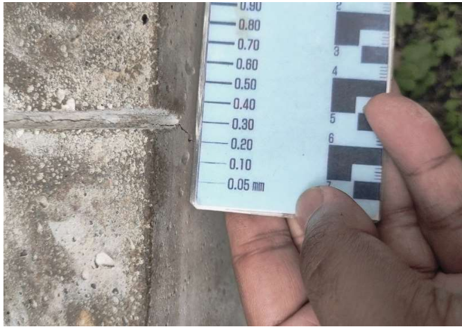
Figure 12: Crack width of 0.2 mm (top view)
