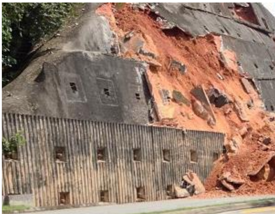
Figure 1: Failure (a) river bank; (b) road embankment and (c) and hill slope (Drdrave,2012) of embankment slopes etc).
