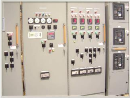
Switchgear: A Necessity for Power Distribution
