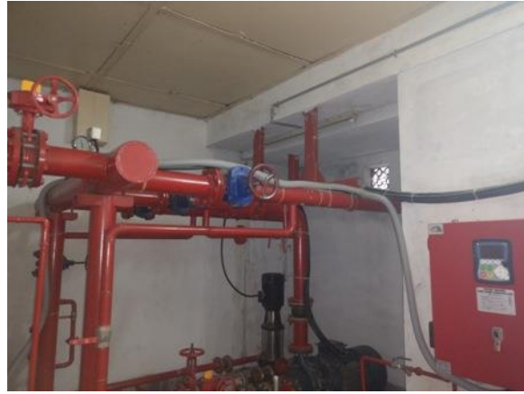
Fig. 5.13: Fire Hydrant System pipe connection
