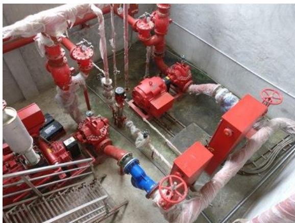
Fig. 5.10: Fire Pump set up
