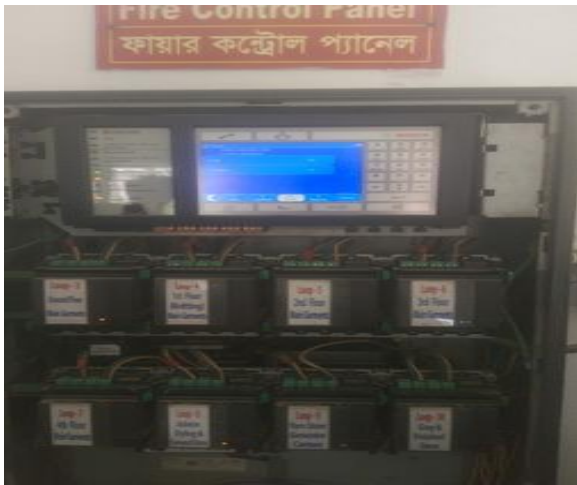
Fig. 5.14: Fire alarm control panel
