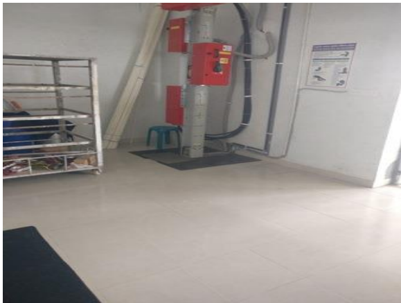
Fig. 5.18: Electrical Bass bar
