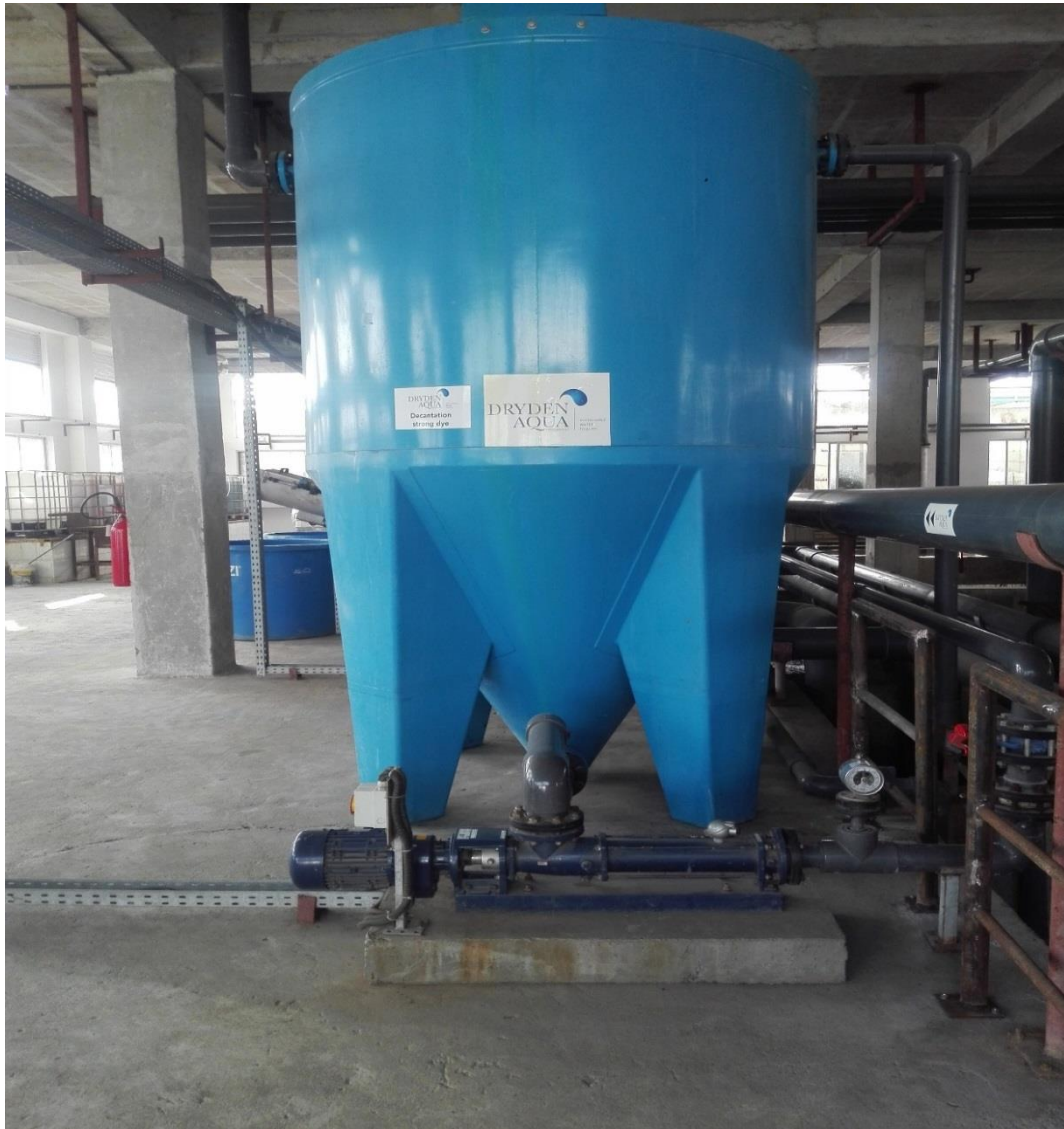
Fig 4.3 Decantation Tank from Dird composite textile Ltd.
