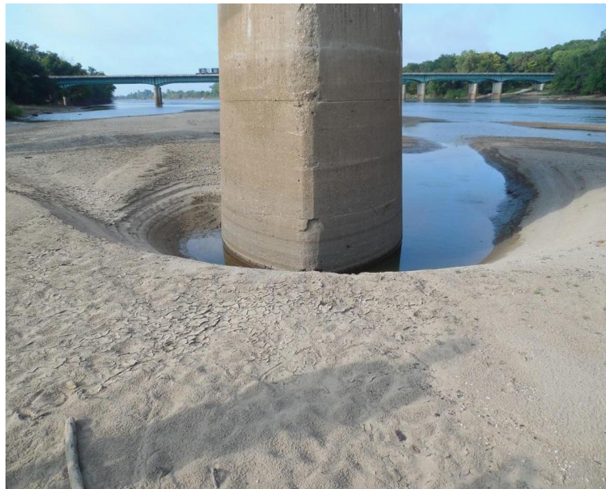
Figure 1: Scouring effect around a bridge pier[16]
