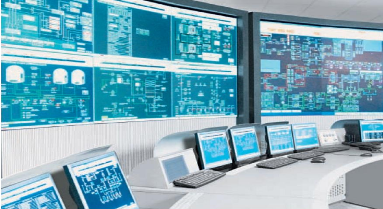
Figure 2.6: Control room for Smart grid system.
