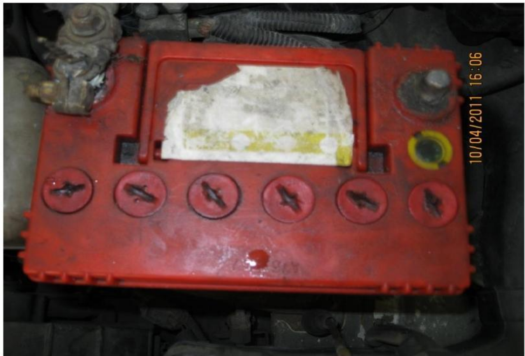
Fig- 2.1 A typical battery for checking for corrosion and cleaning operation
