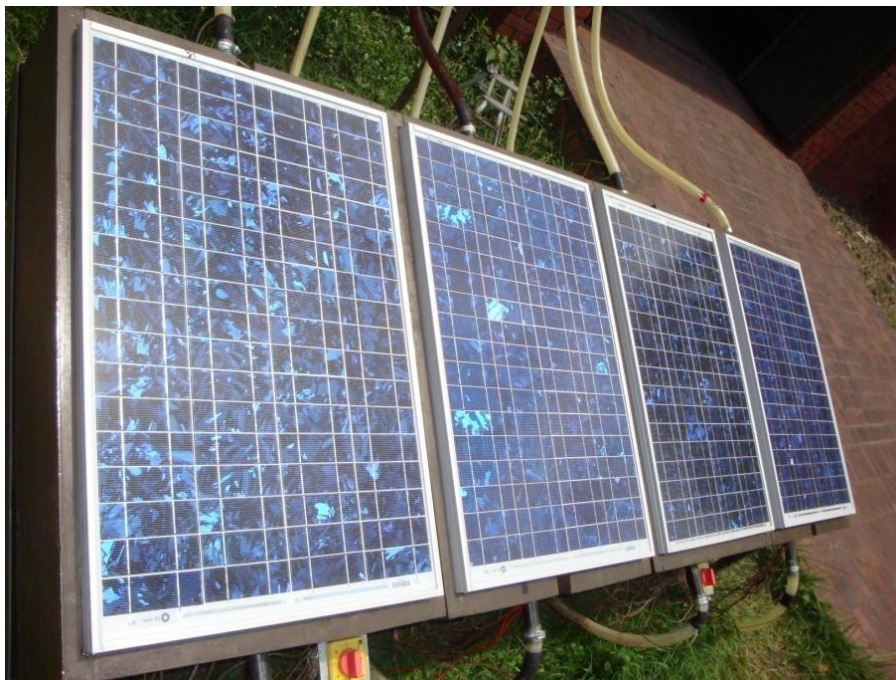
Fig 3.5 Photograph of the installed setup at IUT campus.
