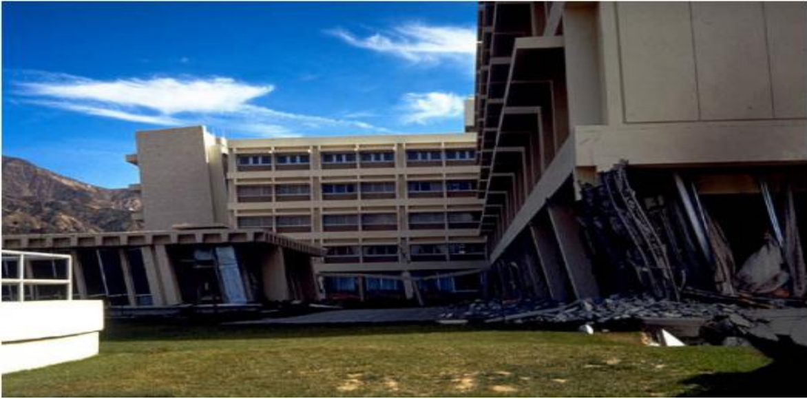
Figure 1.3. Olive View Hospital, San Fernando, California. Partial View of the 5-story Medical Treatment and Care
