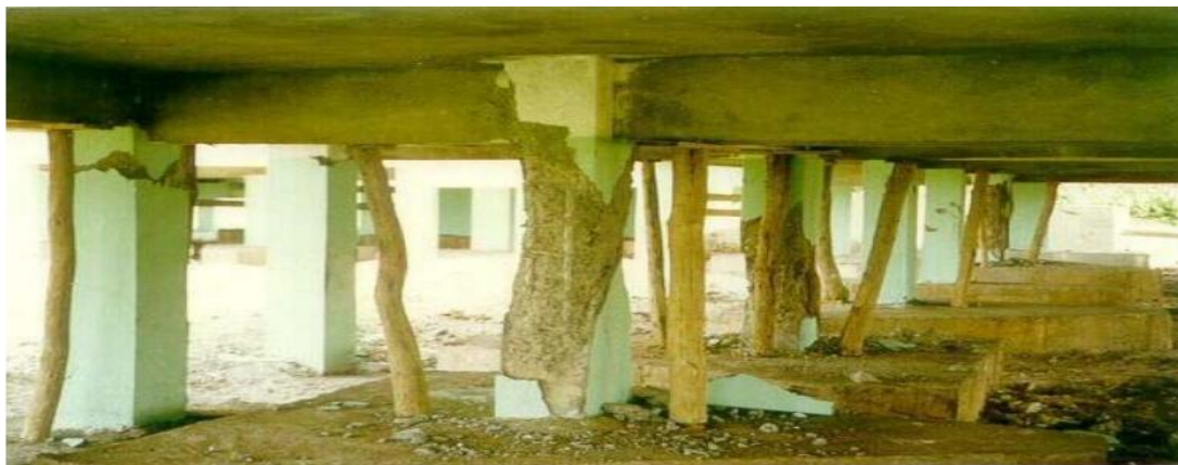
Figure 1.5 Damage to columns in the stilt storey of Youth Hostel building.
