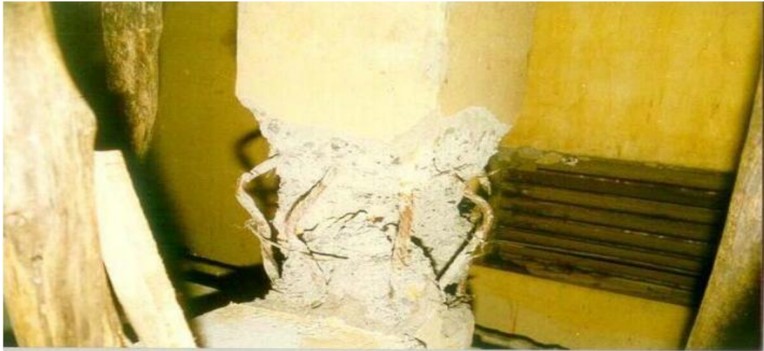
Figure 1.4 Damage to columns in Himgiri apartment.
