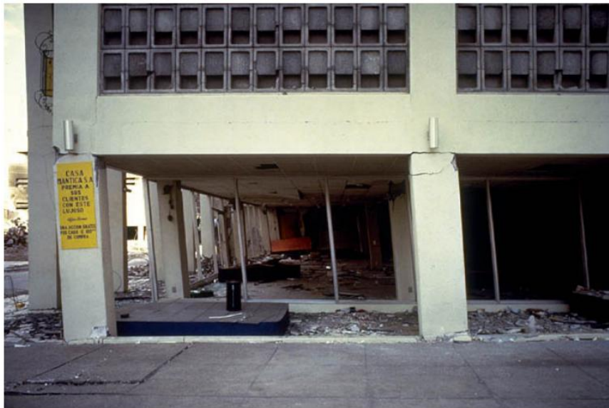
Figure 1.2 Soft-story mechanism in the ground floor in a commercial building during 1997 Managua Earthquake in Nicaragua.
