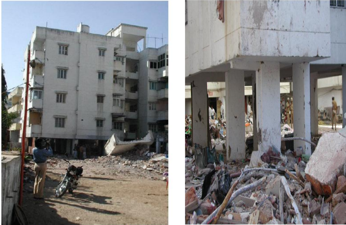
Figure 1.1 Collapse of structure due to earthquake
